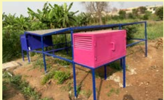
Fixed Mount Structure for Solar System
